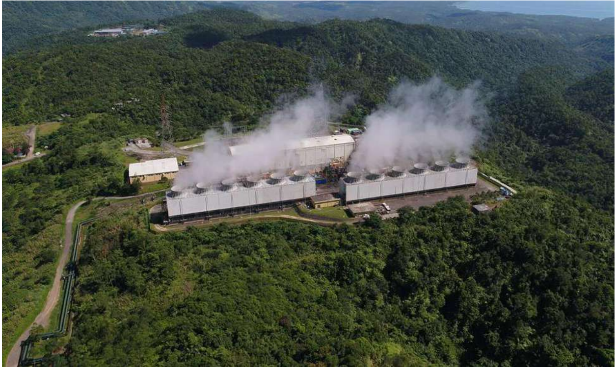
TANAWON GEOTHERMAL POWER PLANT – SORSOGON
