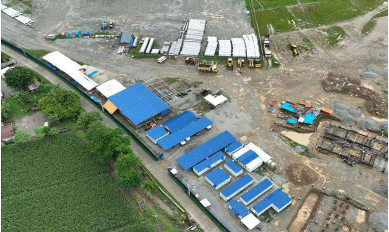
PANGASINAN SOLAR POWER PLANT – PANGASINAN
